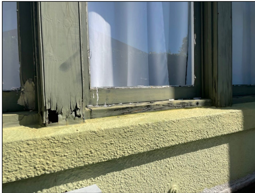
Figure 4: Windows that show some water intrusion and rot on the bottom sill and window casing. Poorly conducted repairs are visible in the bottom corner of the sash on the left.
